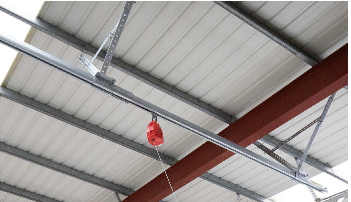
An example of a finished parallel installation.
