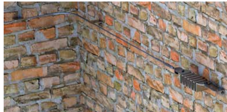
Figure 24 - KeeLine® fitted to Postanka
