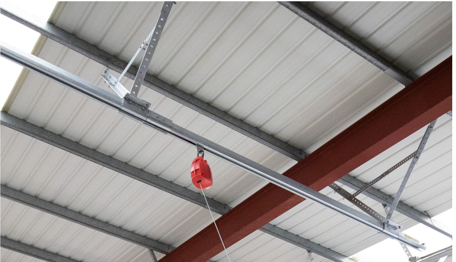
An example of a finished parallel installation.
