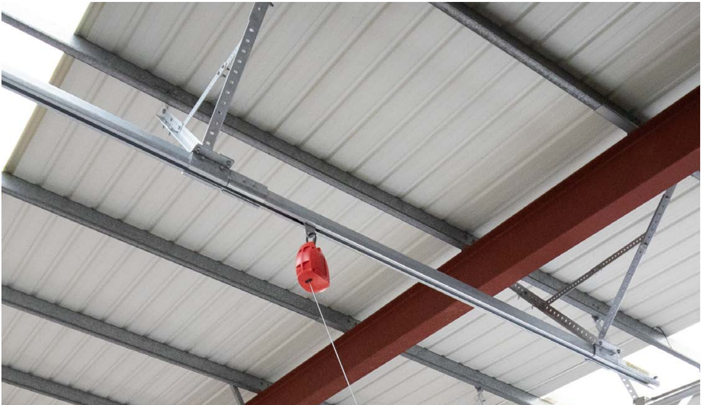
An example of a finished parallel installation.
