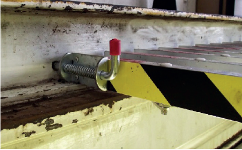
Horizontal spring-loaded pin in hole in pit side rail.
