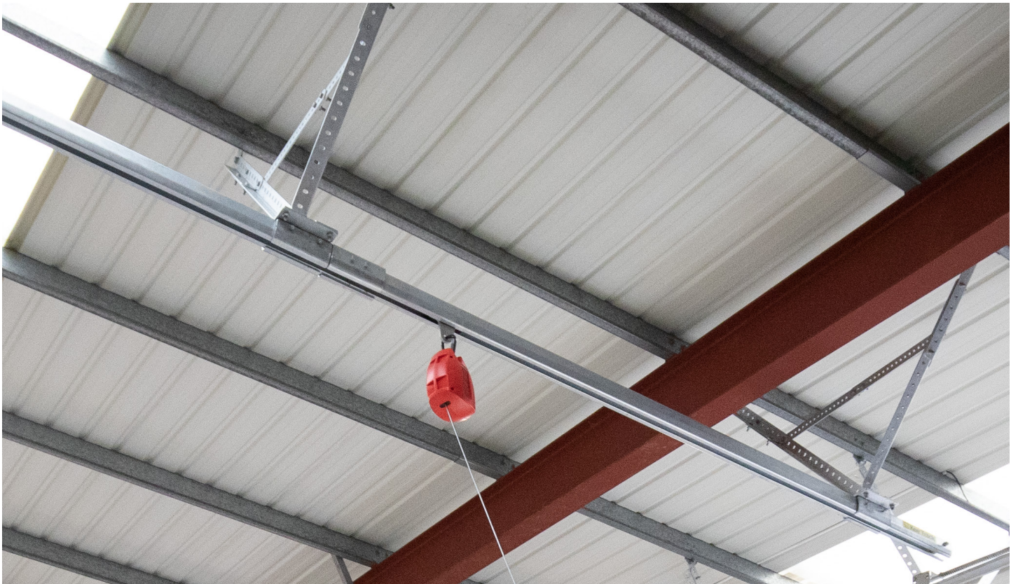
An example of a finished parallel installation.
