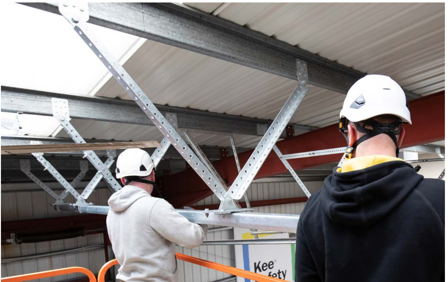
Two installers using an elevated platform secure the rail to the roof infrastructure.
